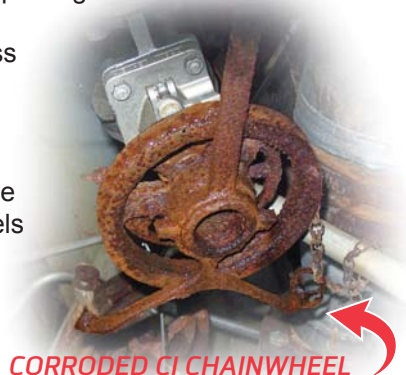
CORRODED CI CHAINWHEEL shows advantage of stainless
